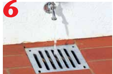
6 Ensure finished surface is 1/8" higher than the grate to assist water drainage.
